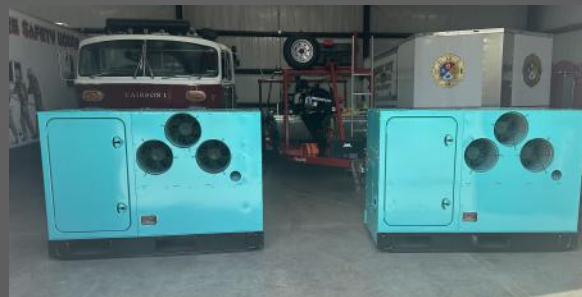
Completed Project Both Generators will replace current Auxiliary Generators at both Station 13 & 19
